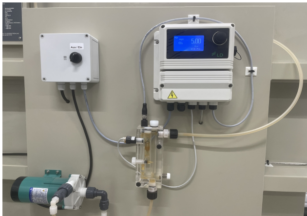
Measurement equipment in a real water installation
