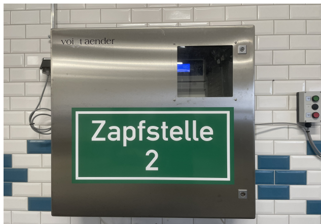
Real potable-water filling infrastructure
